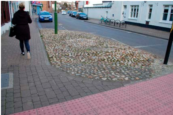
Raised cobbles to control pedestrian movement cause an uncomfortable surface to walk on a dangerous a trip hazard.
